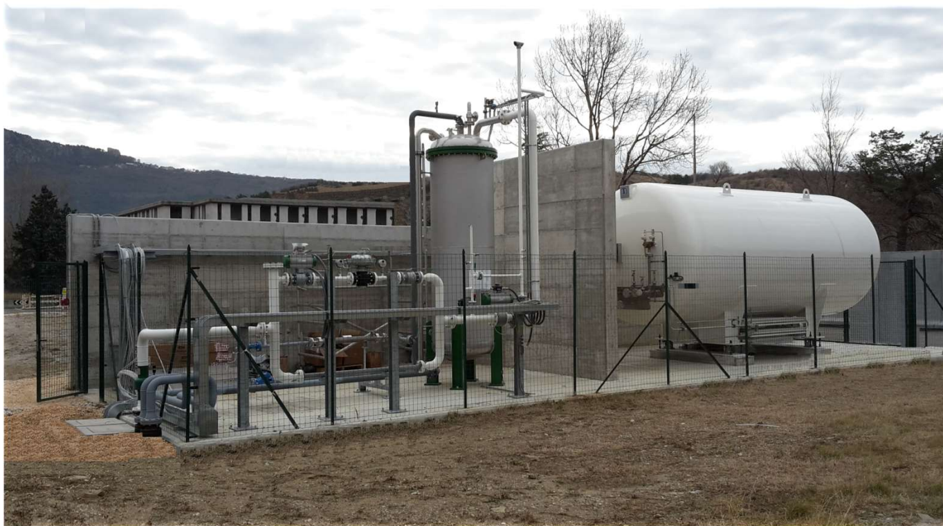
Ethane storage and vaporization plant – Trieste - Italy
