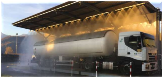
Testing a sprinkler system on a loading/offloading bay
