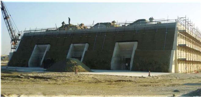
Primary LPG storage - horizontal buried tanks – Venice - Italy
