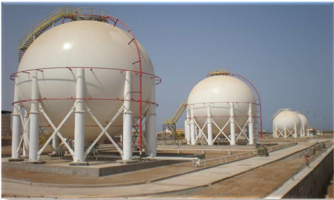
Primary LPG storage - spherical tanks – Massawa - Eritrea
