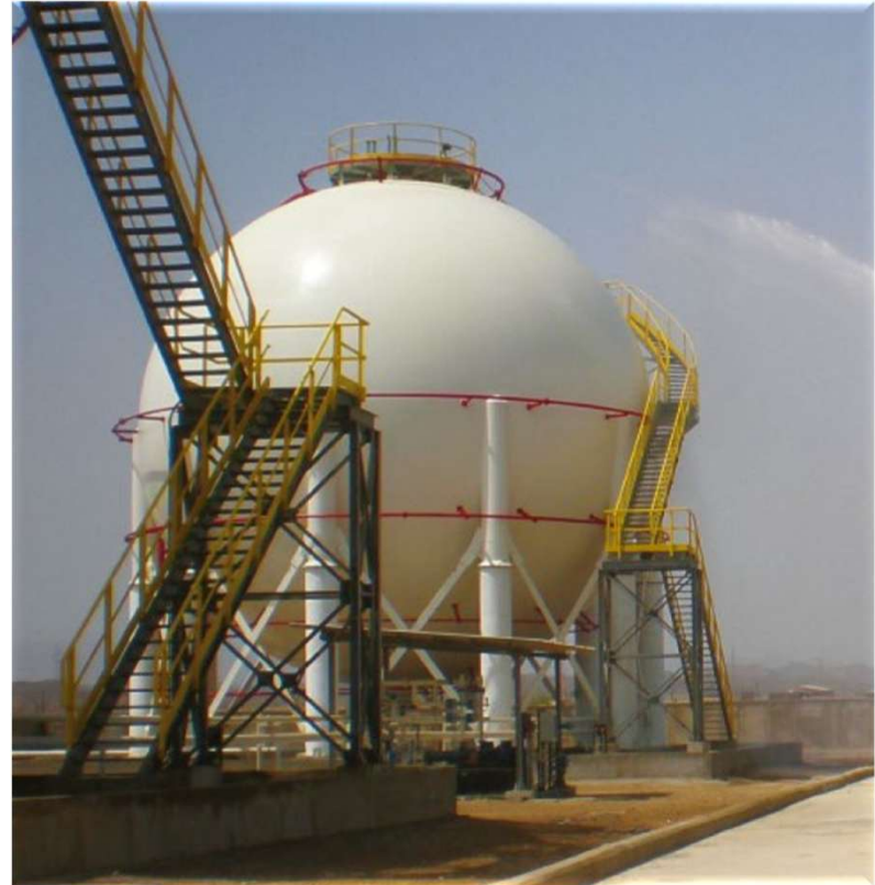
Test of a water monitor on a spherical LPG tank
