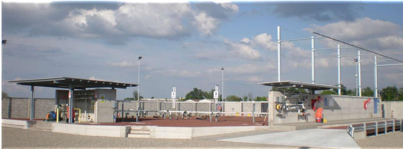
Secondary LPG storage – LPG loading/offloading point and pump room
